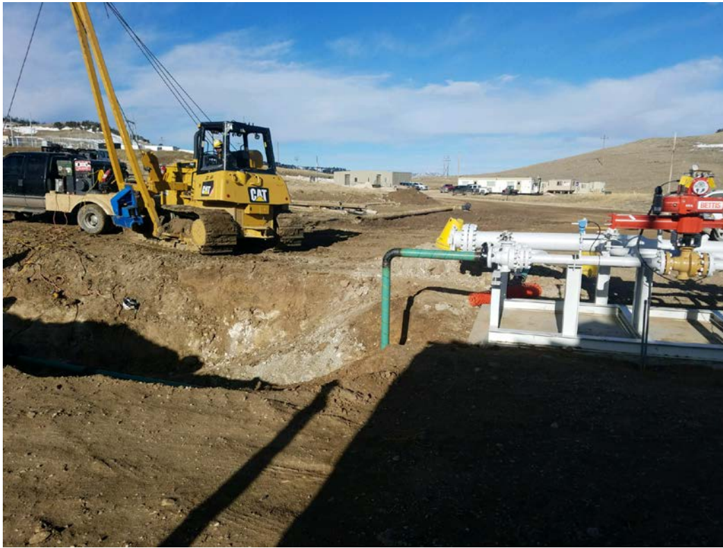
Completion of final connection of Grieve Central Production Facility oil storage and oil sales meter to Grieve Crude Oil Export Pipeline to Casper, Wyoming – March 15, 2018
