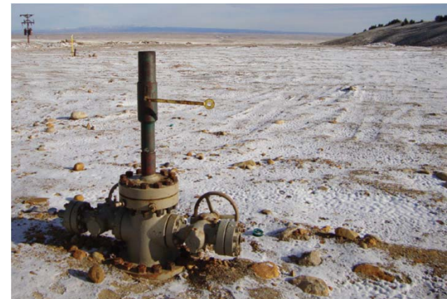
Suspended Grieve 39A well
